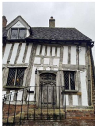
The images left show the street elevation defective panels marked with red crosses, the panels removed, and the finished work.
