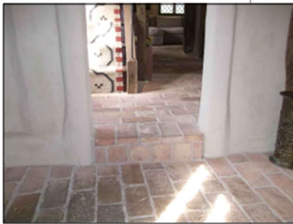
New limecrete floor and underfloor heating with clay brick finish in place of existing concrete floor shown thus
