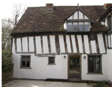
The images left show the rear elevation defective panels marked with red crosses, and the finished work.
